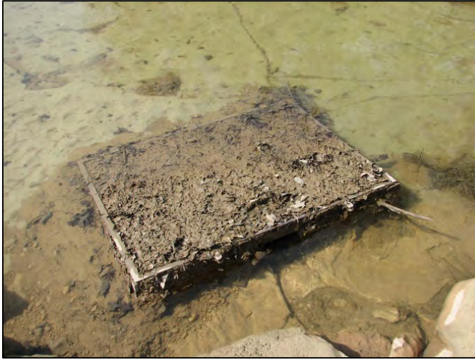
Figure 5. Example of swallet grate with fine debris cover after storm event and prior to manual cleaning.
