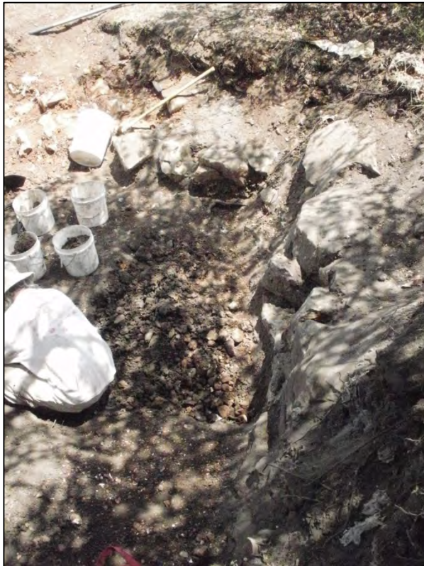
Figure 9-3. The smooth walls of the sinkhole were exposed, demonstrating the feature was actually a trash filled sinkhole. In this case, excavation allows a more definitive evaluation of the sinkhole in addition to removing potentially toxic waste materials.
