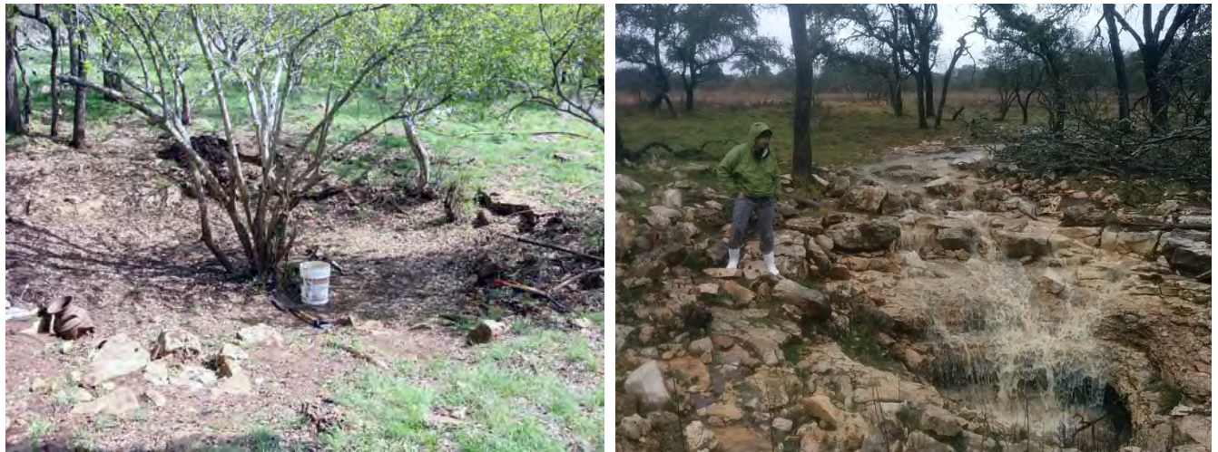
Figure 1-1. (Left) Redberry sink before restoration. (Right) Redberry sink or Possumhaw Cave after restoration on January 22, 2015. Photo by Hanna Morgan, Hill Country Conservancy.
